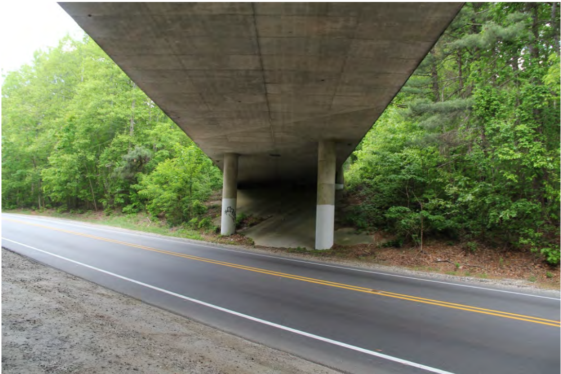
Blue Ridge Parkway, bridge over Sweeten Creek Road, underside, view to southwest
