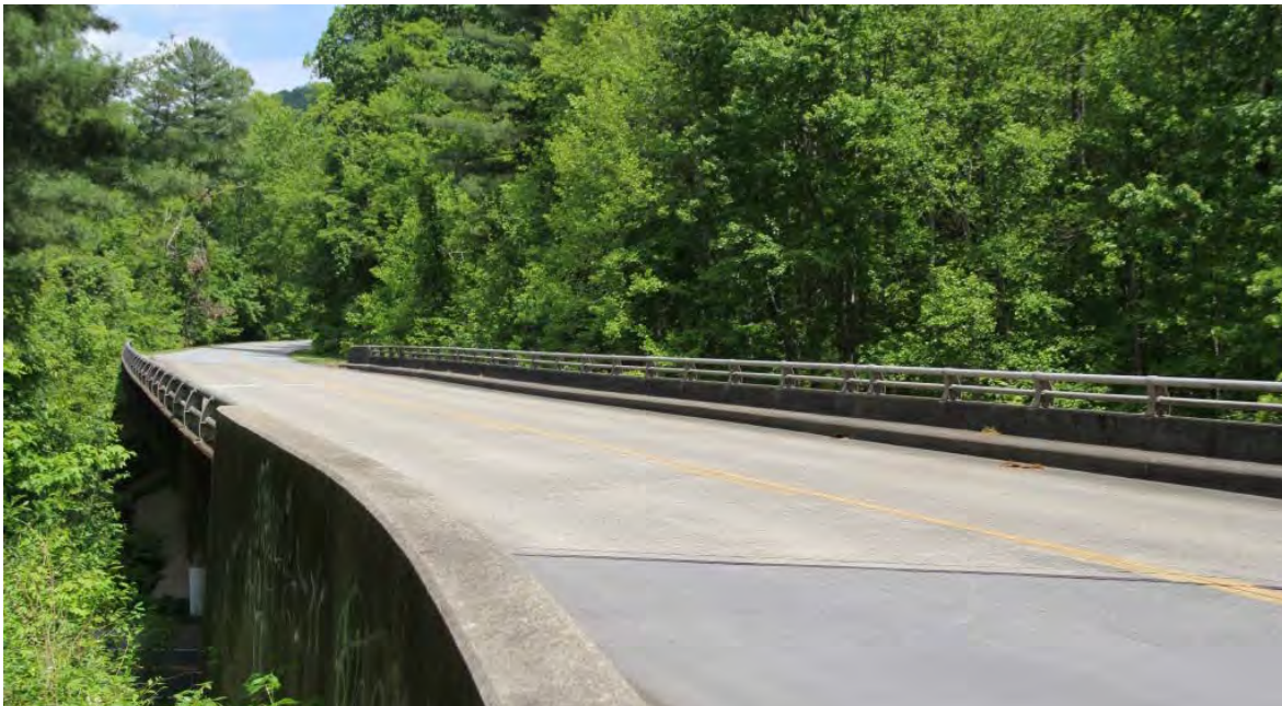
Blue Ridge Parkway, bridge over Sweeten Creek Road (US 25A), view to east
